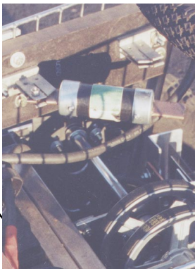
Combined fuse and knife switch.
